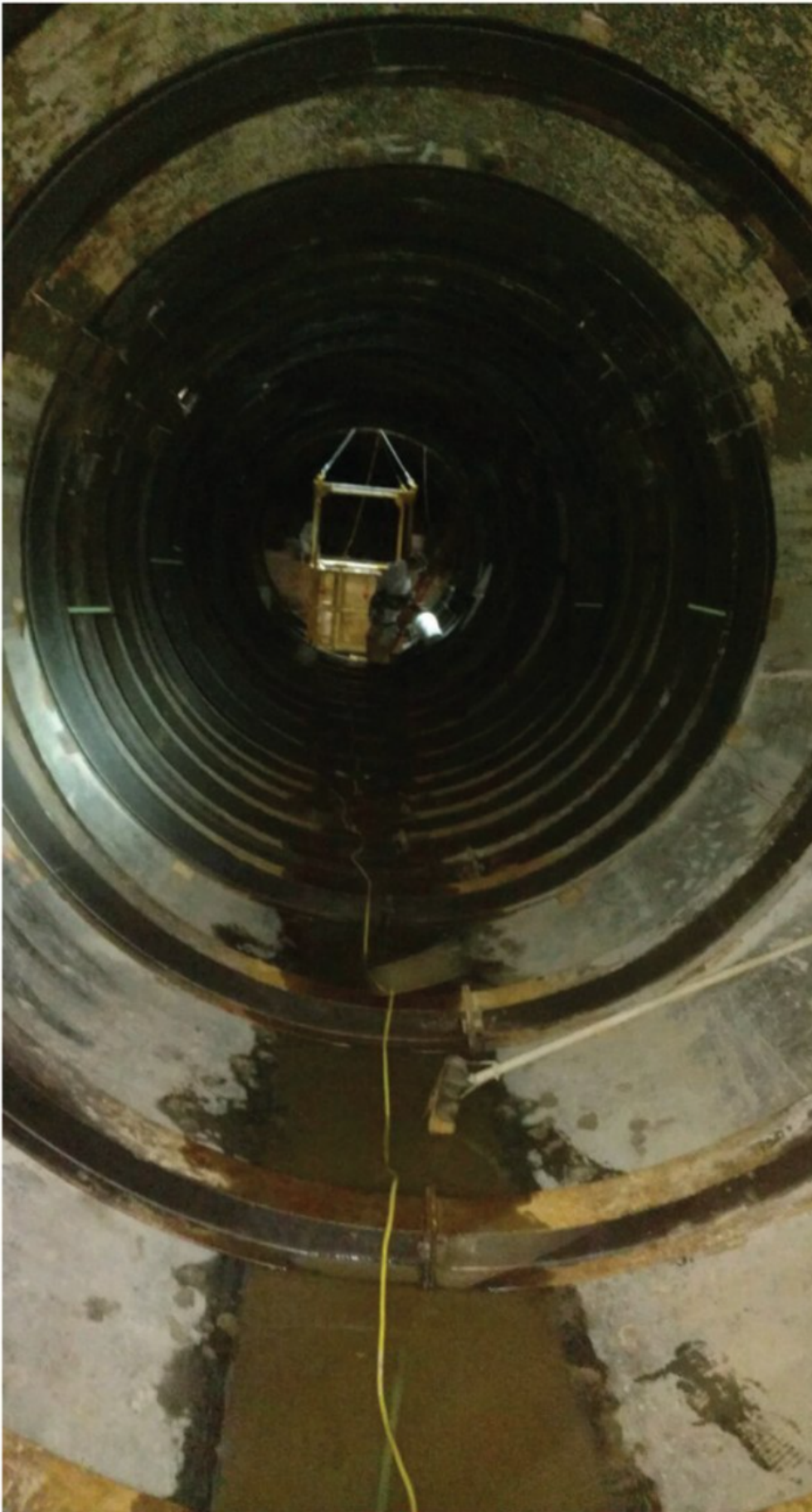
Metal ribs were installed in the pipe adjacent to the collapsed interceptor. Once the pipe was pumped out, cleaned, and inspected, it was found to be riddled with cracks and leaks. It will be lined as part of the repair process. About 1200 m (4000 ft) of the interceptor – the collapsed portion and another 1128 m (3700 ft) deemed to be in imminent danger of collapse – will either be replaced or lined with fiberglass polymer pipe. Macomb County (Mich.) Public Works
