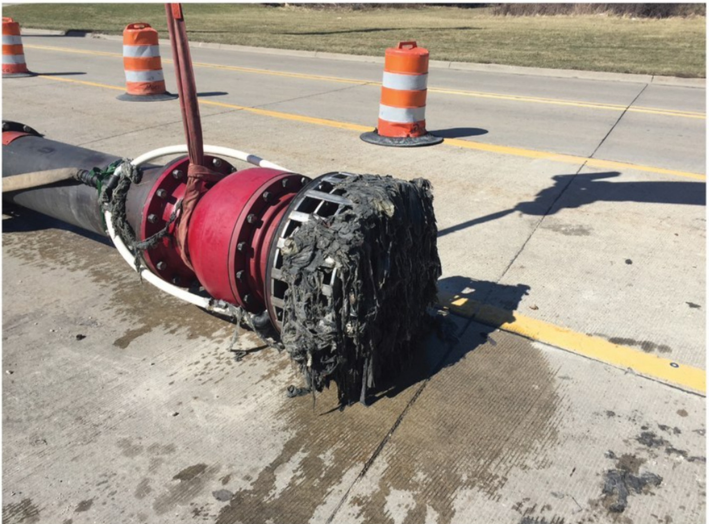
During this massive bypass-pumping project, pump clogs caused by ragging were an issue. Macomb County (Mich.) Public Works
